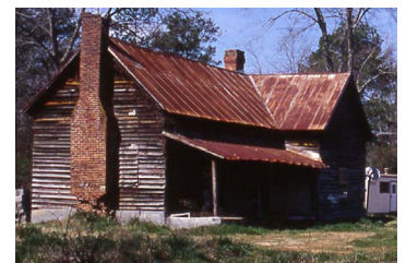
This gabled ell residence is located on Saffold Road. Photo by Tiffany Tolbert
